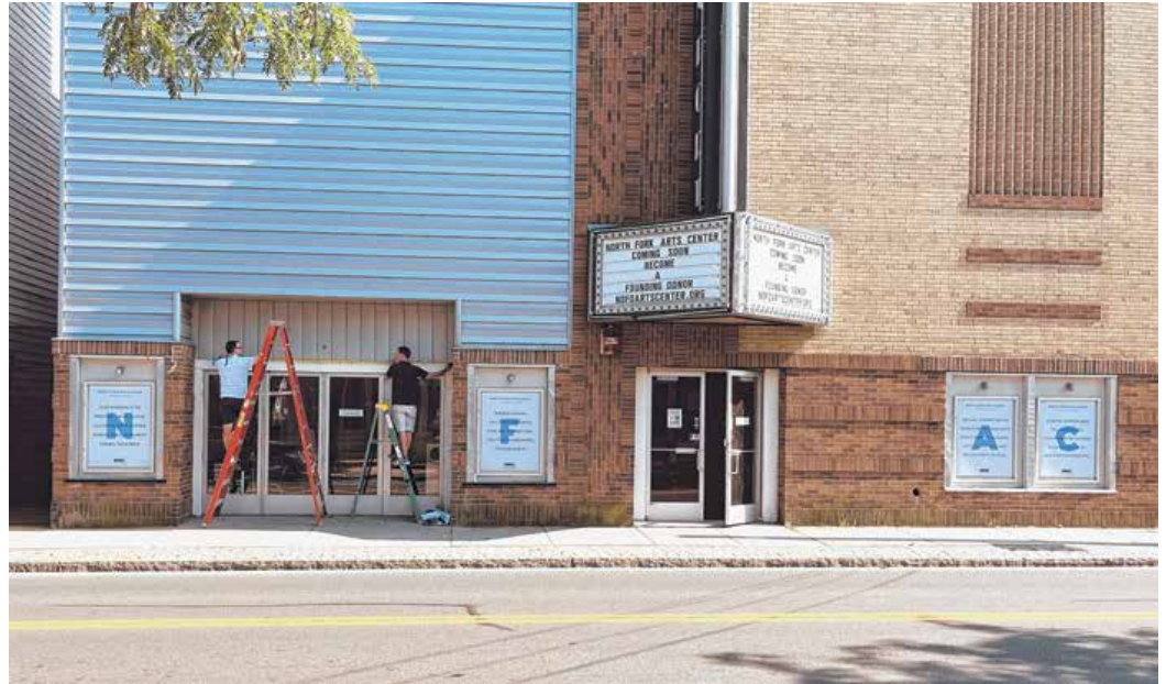
THE NEW TEMPORARY SIGNAGE IS UP, SIGNALING THE MOMENTUM BUILDING BEHIND THE NFAC'S DOORS.
